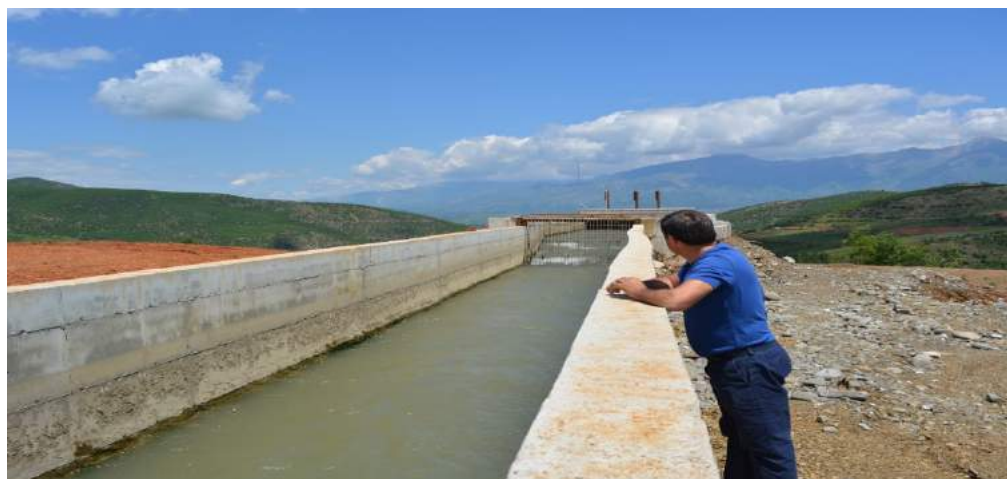
Small Hydropower Plant in Librazhd, Albania.
