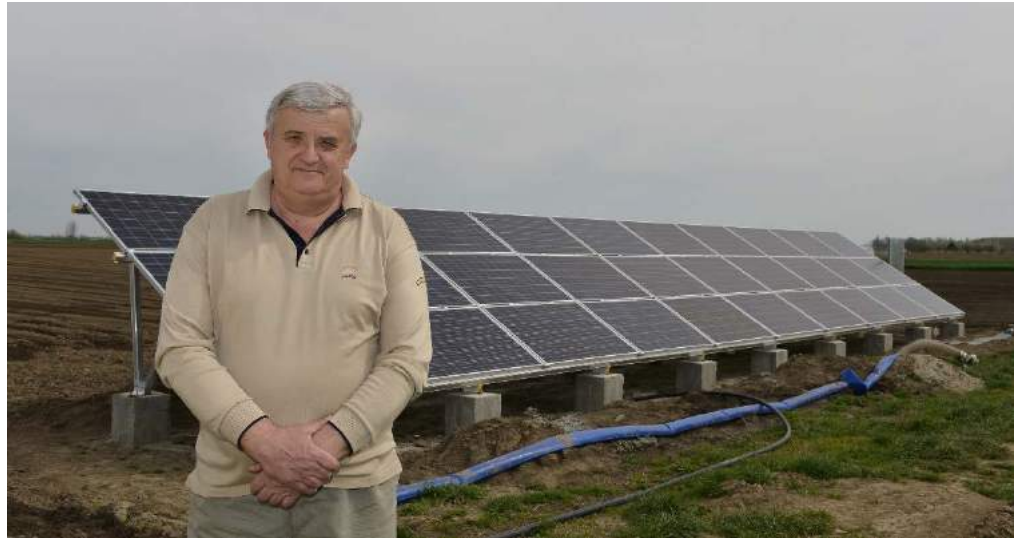
Solar-powered Irrigation Drip System in Begeč, Serbia.
